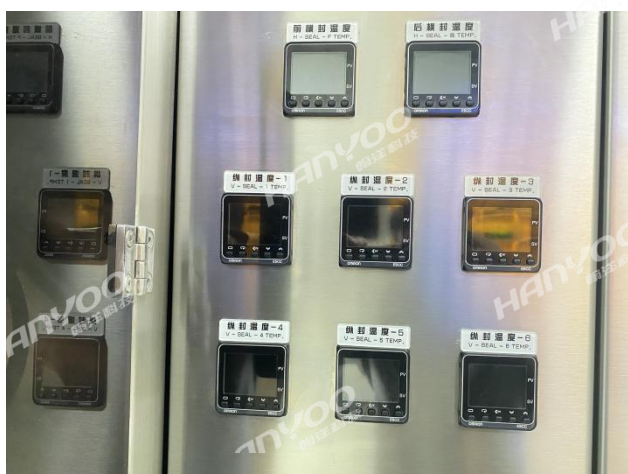
Temperature control pane
