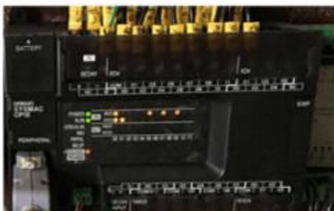
Japan Omron PLC Control System
